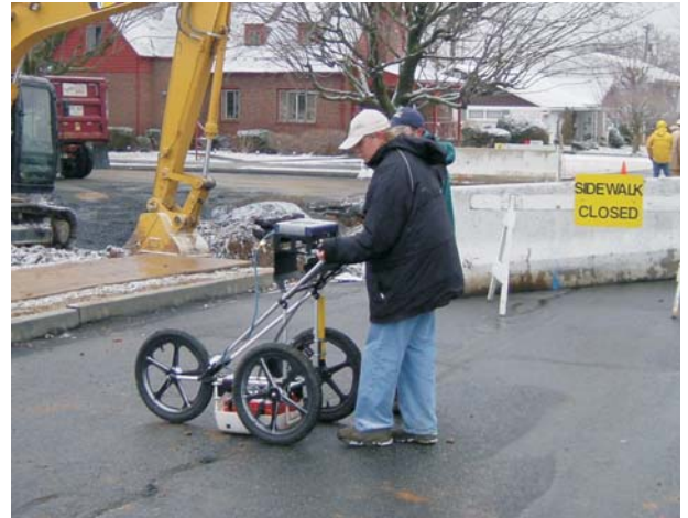
ARM Geophysicist scanning with GPR for subsurface voids and potential collapse features.
